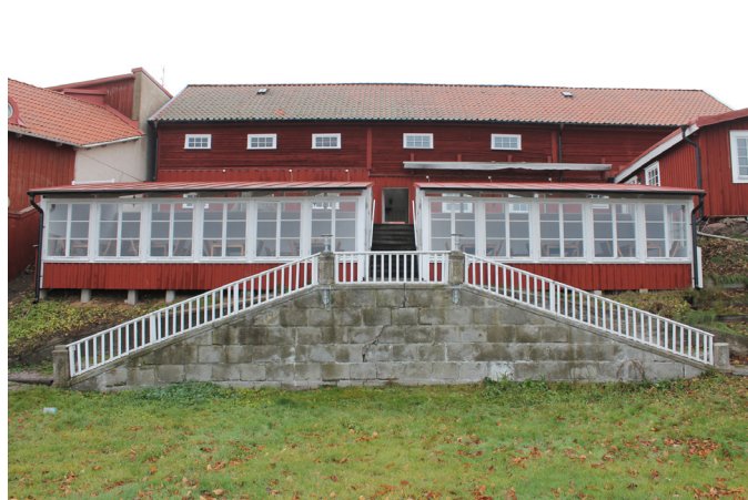
Topography slopes down to the backyard. On the slope, there are two small non-insulated rooms that were added in 2004.
