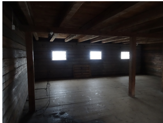
The right room of the building was not used and it does not have interior cladding.
